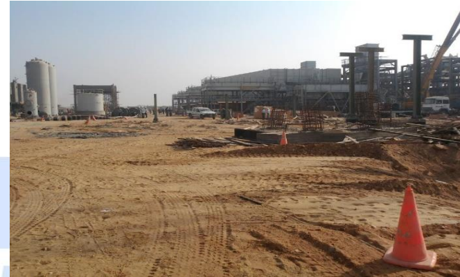
DAHSOUR COMPRESSOR STATION
